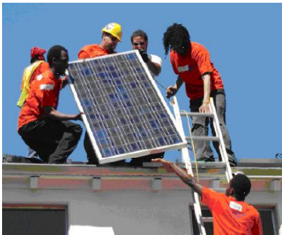
Richmond BUILD program graduates install solar panels on the home of a low-income Richmond resident. Along with its solar partners, Solar Living Institute, Solar Richmond and GridAlternatives, RichmondBUILD prepares trainees to be tomorrow's green-collar workers in the solar industry. Richmond BUILD also prepares their students for the construction industry as well. Source: RichmondBUILD
